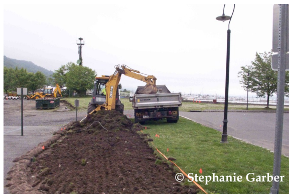
Village of Piermont Highway Department at work removing excess turf and soil
